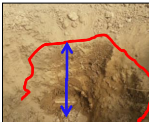
Figure 2: Dry soil surface over the irrigation pipe
