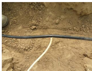
Connection with the submain line (PE pipe Ø 17 mm)
